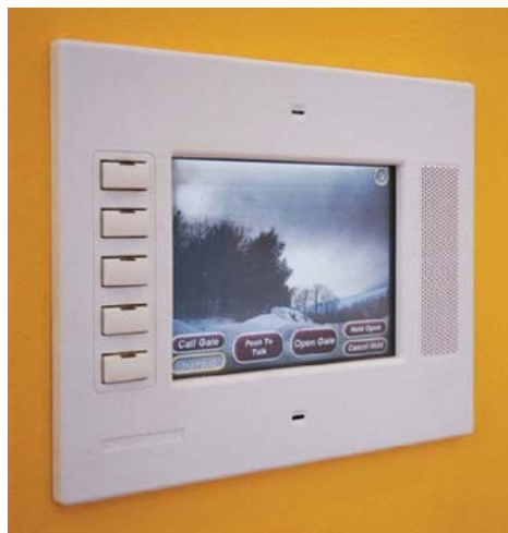
A Crestron touchpanel shows the gate control screen with video from one of the home's outdoor cameras.
