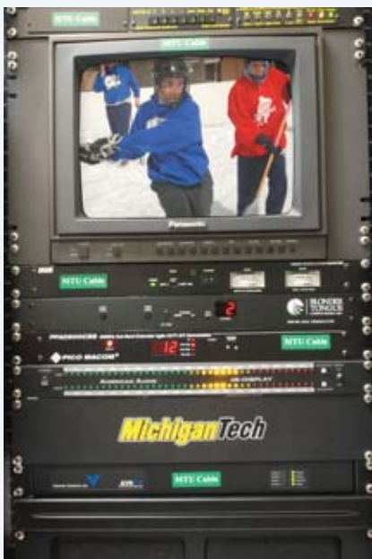
An AVN210 encoder in one of Michigan Tech's data centers, streaming video out to Internet2
