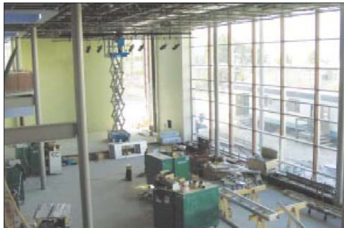
On this design-build job at a community college in Seattle, Delta AV Systems, Portland, OR, installed projection and audio equipment in this multipurpose educational space.
