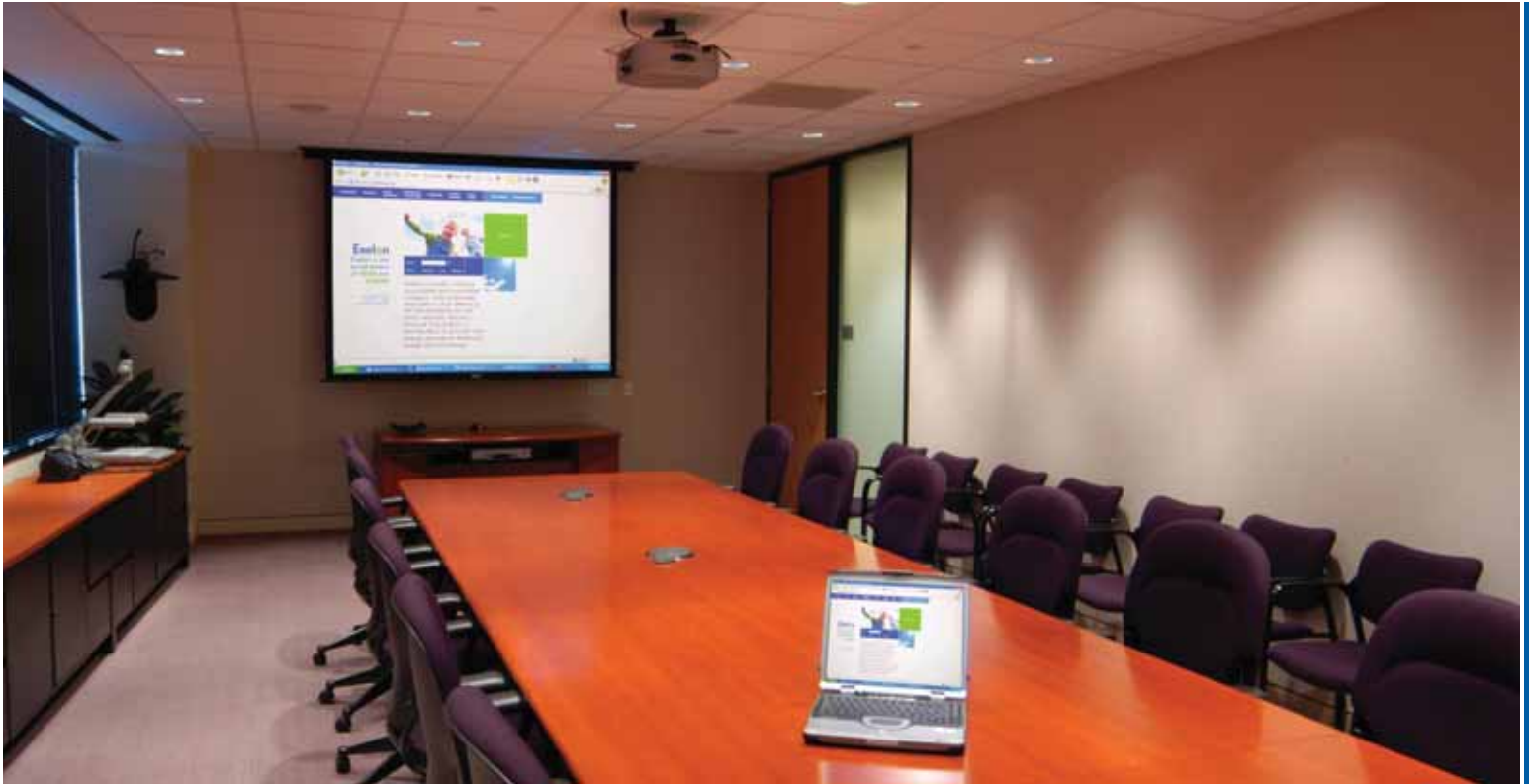
Videoconferencing system in the operations center conference room
