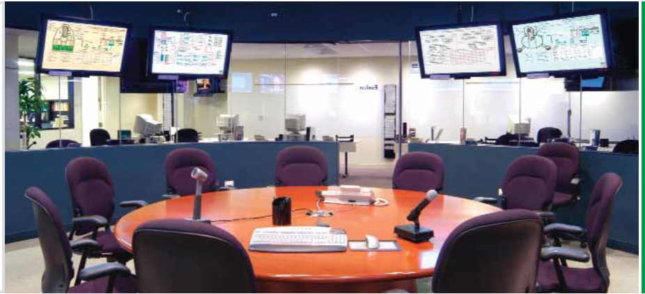
The EOF with four of its eight flat-screen monitors, satellite, radio and telecommunications gear. The training center is show below.
