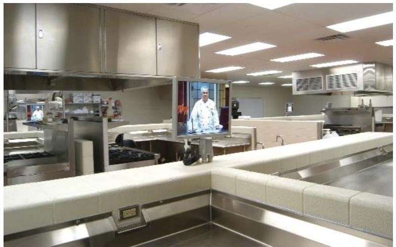
Top: one of the baking classrooms with its projection system. Immediately above: the demonstration classrooms features overhead hood vents for the student cooking workstations, necessitating individual LCD monitors.
