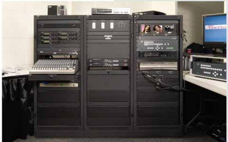
The equipment rack plus a switcher Novatoo added for the annual meeting.
